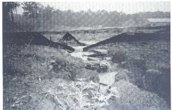
A failing silt fence results in sediment pollution to stream.
